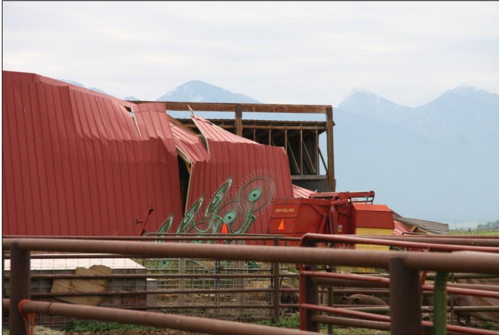
Figure 19 – Structural damage to a metal barn structure four miles west of Pablo, MT (photo courtesy of Bryan Henry).
