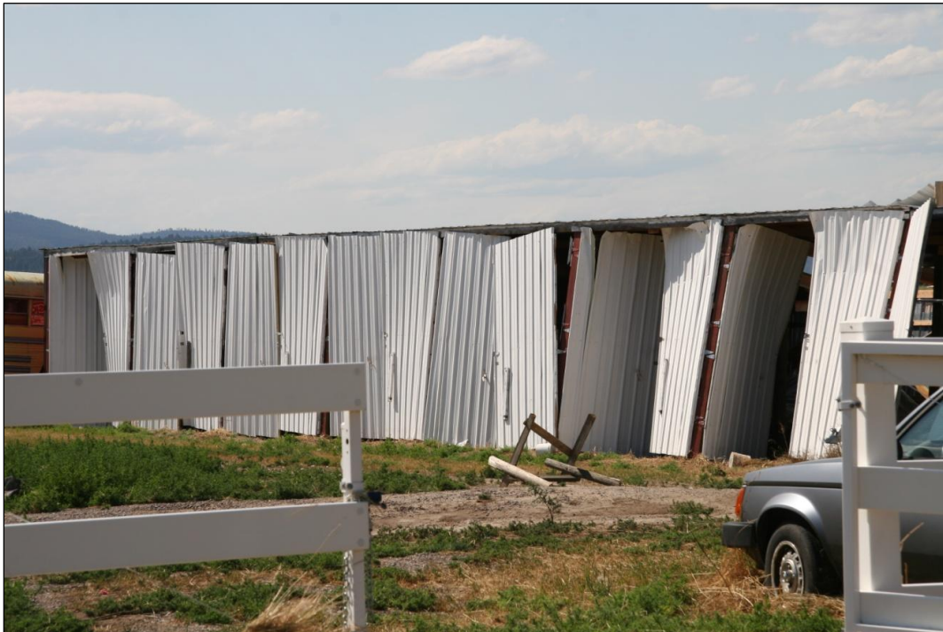
Figure 22 – Structural damage to a metal barn near Somers, MT (photo courtesy of Bryan Henry).
