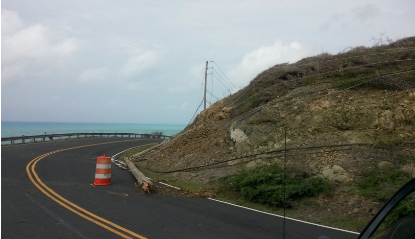
Fig. 19. Broken light pole at Turners Hole and Grass Point on Route #60, St. Croix.
