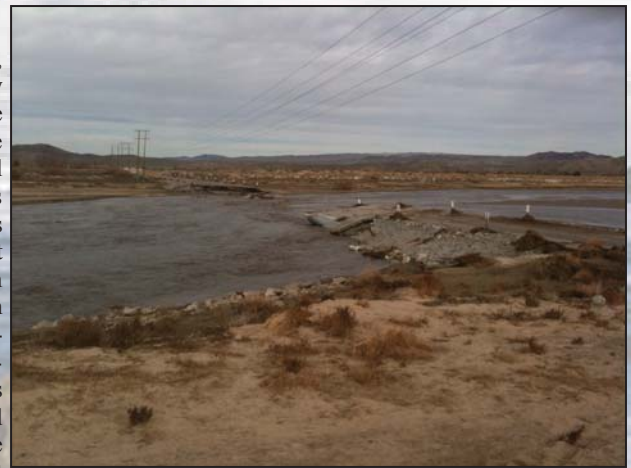
The Mojave River washed out a bridge at Lenwood in December 2012 due to flooding from heavy rain, and snow in the mountains. (Photo: John Fertsch)
