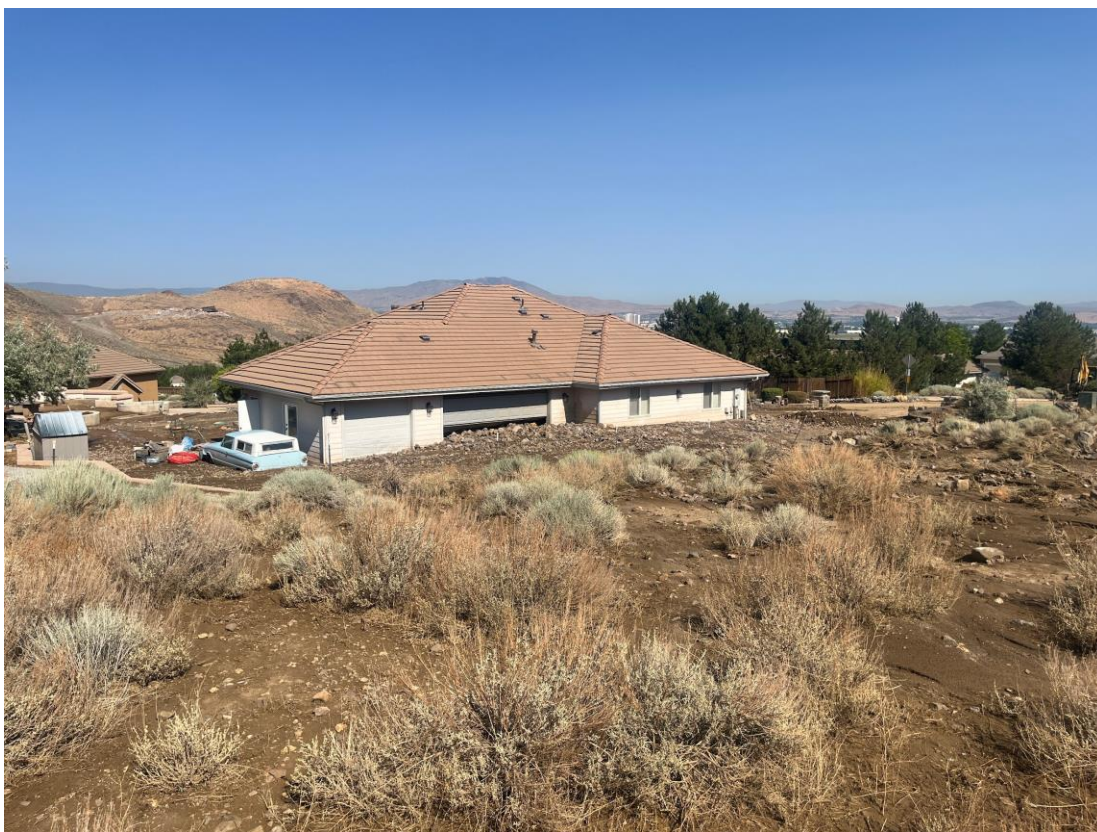
Photo 3: Image of the most severely damaged home from the Hidden Valley flooding on July 21st. More common impacts included mud and debris on landscapes, driveways, and roads.
