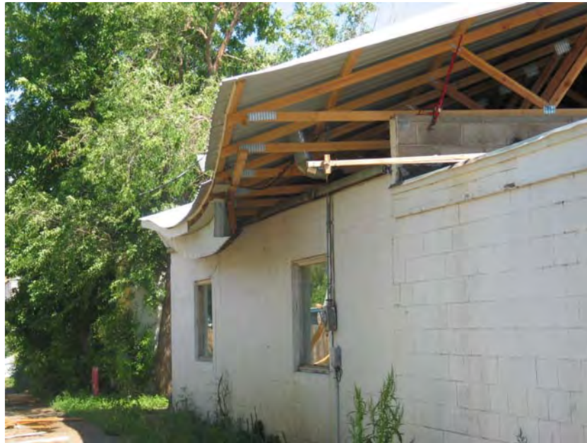
Wind damage to the roof of a business. The damage was typical of what was observed in Glendive by the National Weather Service storm survey team.
