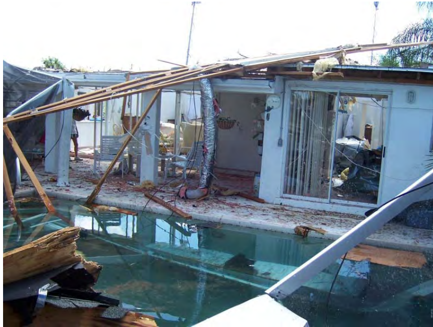
A well anchored roof was ripped off this home and roof debris was found a half mile away impaled in the ground. Photograph by Daniel Noah, National Weather Service, Ruskin, FL.
