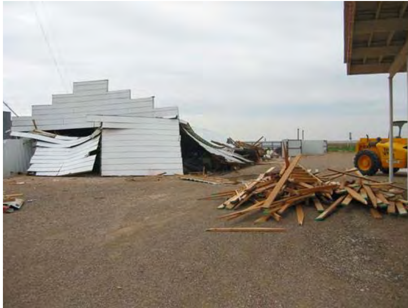
A heavily damaged industrial barn and scraps of lumber gathered by clean-up crews compose this scene following thunderstorms that produced significant wind damage in the Anton vicinity of northeastern Hockley County during the early evening hours of the 3rd. Damages there exceeded $400,000. Photo courtesy: National Weather Service - Lubbock, Texas.
