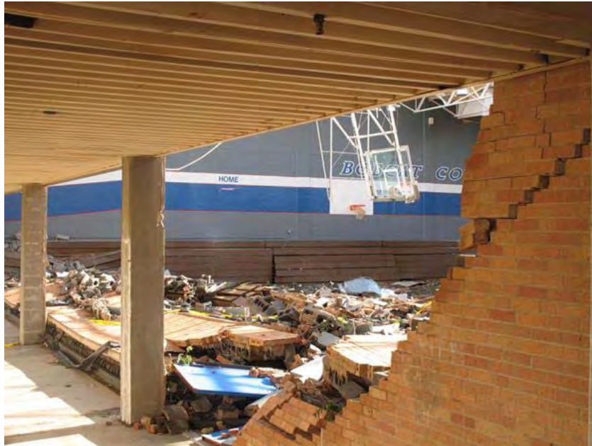
The Childress High School suffered a direct strike by an F2 tornado during the evening of the 9th. Several million dollars worth of damage was sustained at the school district's facilities. A 109 MPH wind gust was recorded as the tornado moved across the campus. The gymnasium (pictured above) was destroyed. Photo courtesy: National Weather Service - Lubbock, Texas.
