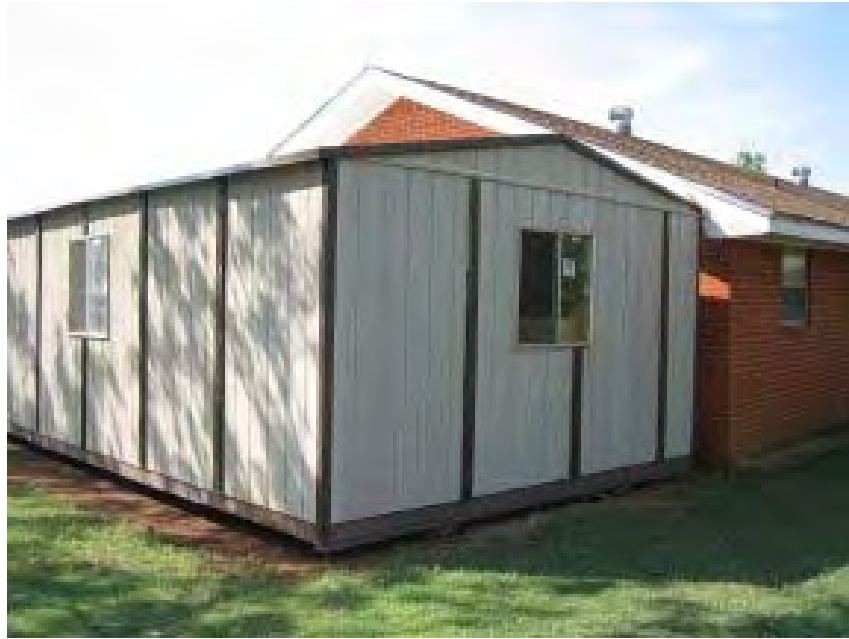
Looking closely at the picture, one can see that the shed has been moved about a foot and a half towards the house, stopping only after it hit the house. Photo courtesy: NWS Midland Damage Survey Team
