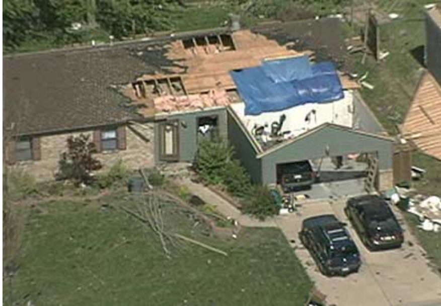
An aerial view of a home damaged by the tornado in Shiloh, IL.
