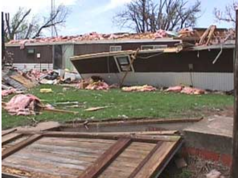
Trailer house damaged by tornado approximately 2 miles southwest of the intersection of State Highway 45 and the Woods County line.
