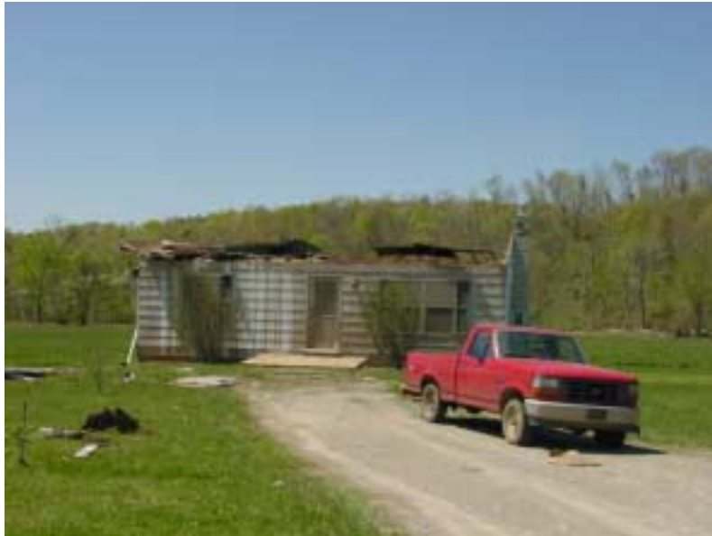
A small home that was severely damaged by the tornado in Madison County, MO
