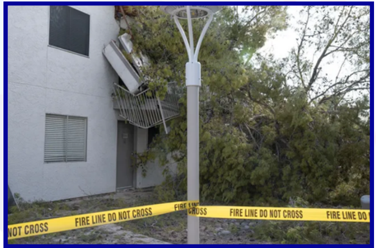
Storm damages at Avia McCormick Ranch Apartment Homes. Photo by Mark Henle/The Republic
