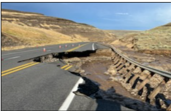
Highway 2 Washout in Douglas County July 2023
