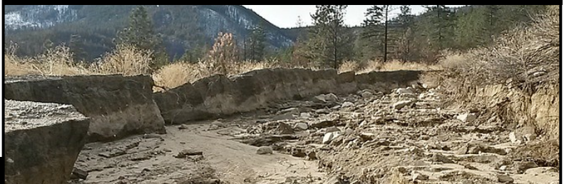
Flooding on Black Canyon Rd in Okanogan County—courtesy Omak Chronicle—11/17/15
