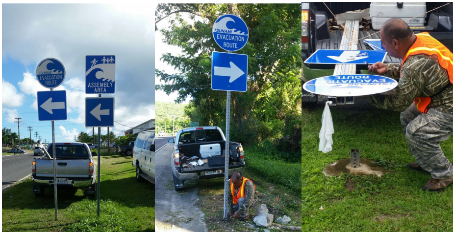
CNMI HSEM staff do quarterly island-wide assessments of tsunami signs to ensure signs have not been tampered with or altered. If necessary, signs are removed for cleaning and then reinstalled
