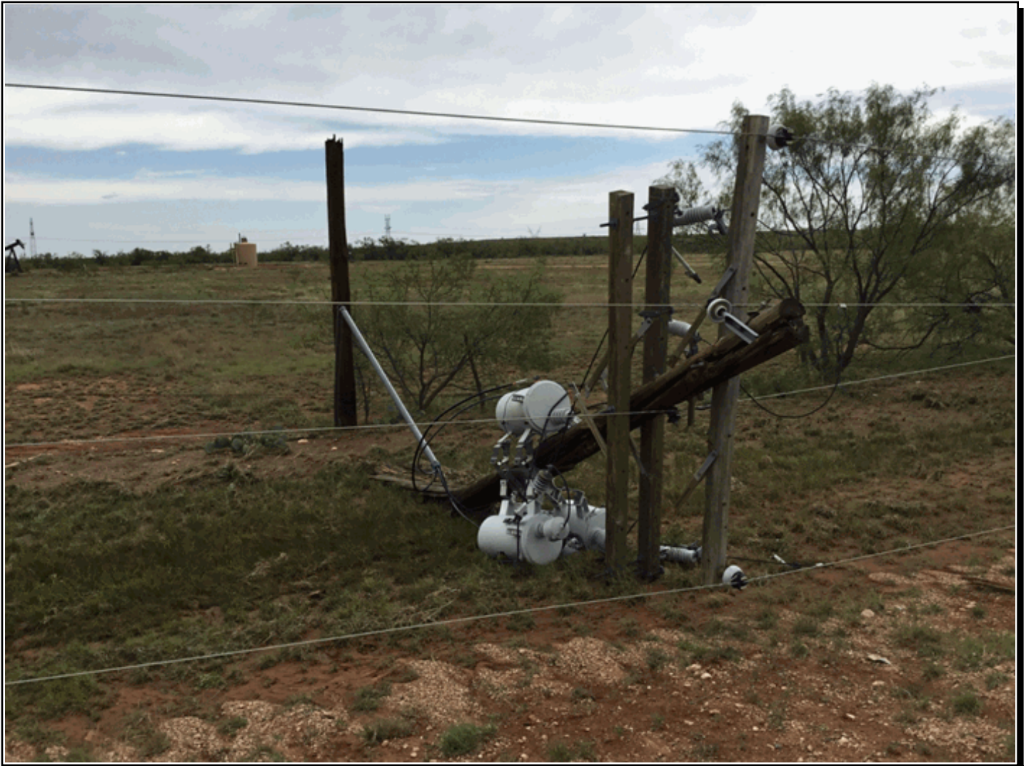
A thunderstorm moved across Scurry County and produced wind damage in the southeast part of the county. Winds around 100 to 110 mph snapped and mangled over 200 wooden power poles. Photo is courtesy of the NWS survey team.
