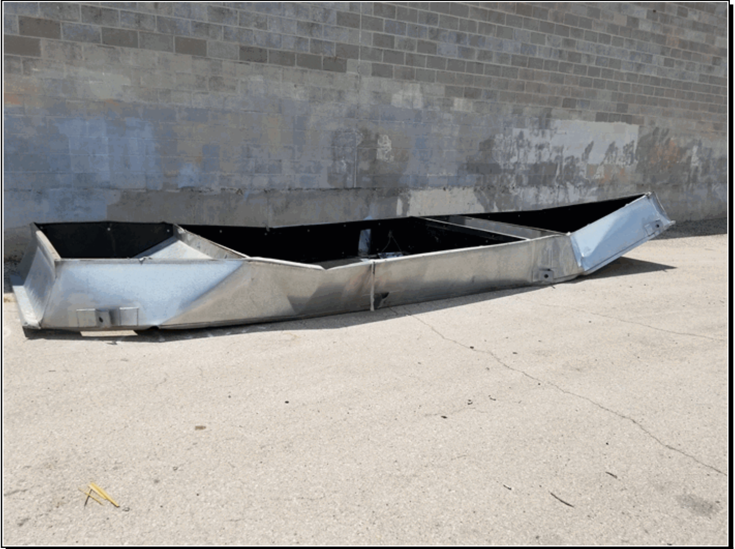
Pieces of HVAC equipment were lifted off the roof of the Albertsons in Hobbs, NM due to thunderstorm winds. Photo courtesy of the NWS survey team.
