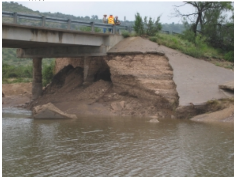
A bridge on State Highway 349 was condemned by Texas Department of Transportation officials after flash flooding along Dry Creek severely damaged the structure early Sunday, July 25th. Over eighteen feet of water raged through the creek and washed away concrete and earthen embankments leaving a single concrete pillar to support the bridge. The bridge's structure also was cracked in several locations. Photo courtesy: National Weather Service - Midland/Odessa, Texas.
