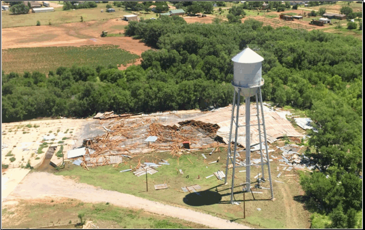
Aerial view of a large warehouse in Turkey, TX destroyed by intense microburst winds. Photo from NWS Lubbock staff.
