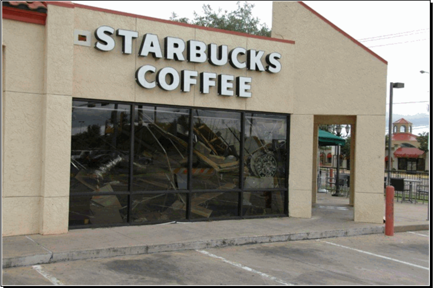
Heavy rainfall and accumulating water atop a flat-roofed structure resulted in the collapse and destruction of a Starbucks Coffee store in Lubbock during the late evening hours of the 3rd. The manager was credited with saving the lives of nearly a dozen employees and patrons seconds before the roof collapsed. Photo courtesy: Bill Hopkins - National Weather Service - Lubbock, Texas.
