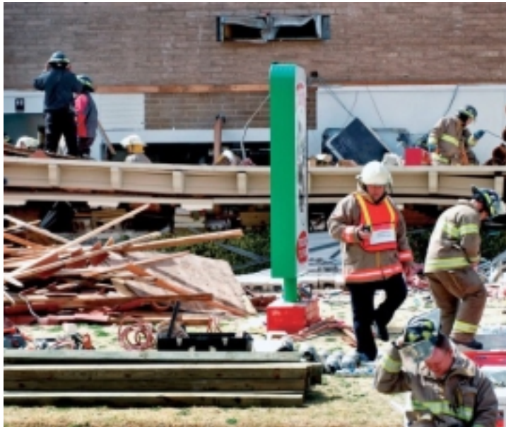
Rescue workers search for trapped victims in the rubble of the Little Panda restaurant after high winds contributed to the building's collapse. One woman died and nine people were injured when a sign was blown down and caused the roof of the structure to fail. Photo courtesy: David Johnson - The Daily Toreador.
