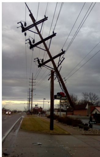
Above: Power pole snapped in half along Watson Road in Crestwood
