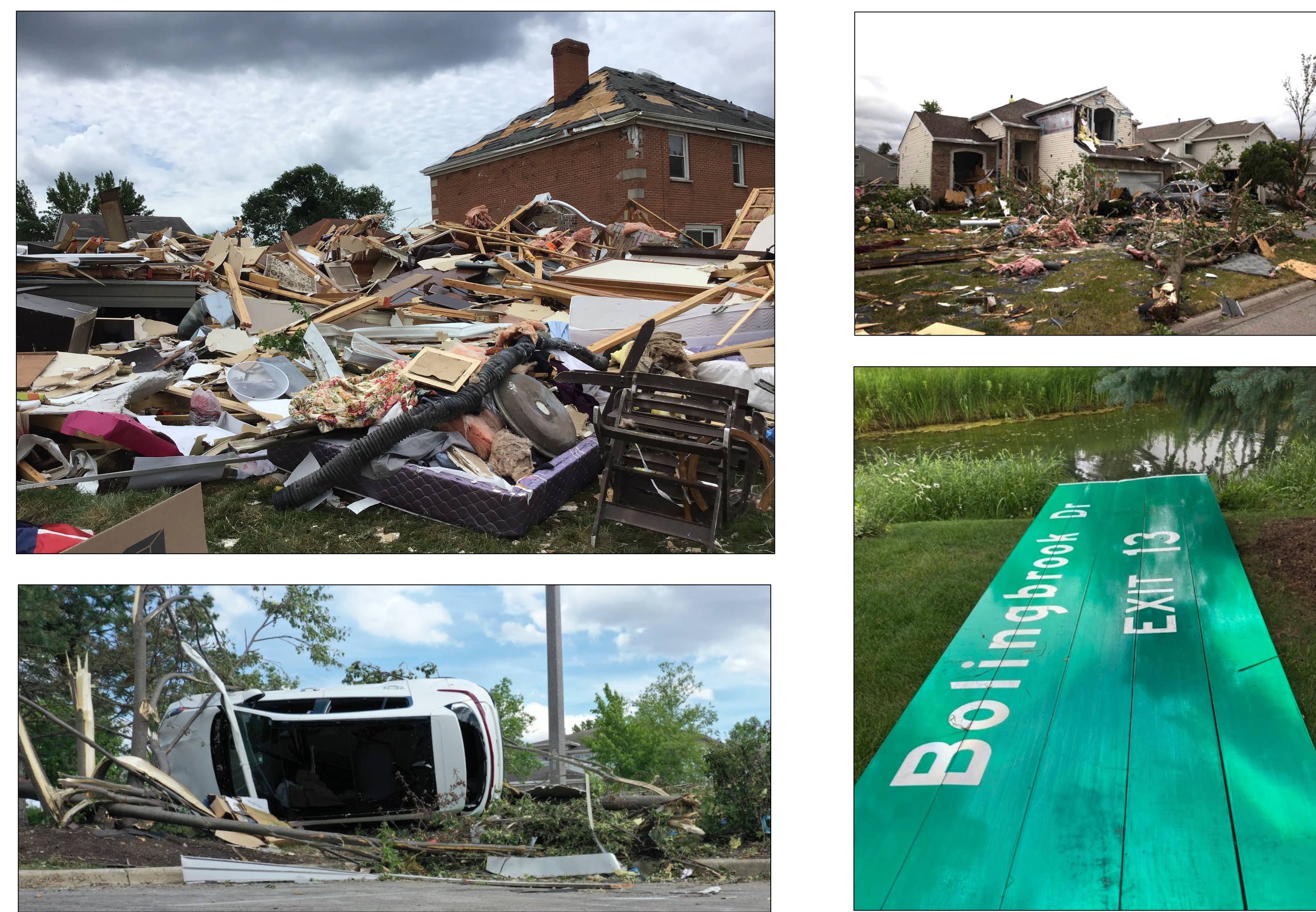
Figure 2: Photos from damage surveys conducted by NWS Chicago and the University of Illinois Wind Engineering Research Laboratory. Upper left: Destroyed home in Naperville where tornado was peak intensity. Lower left: Vehicle rolled in Woodridge. Upper right: Home damage in Naperville. Lower right: I-355 exit sign that was tossed 6 mi. (~9.7 km).
