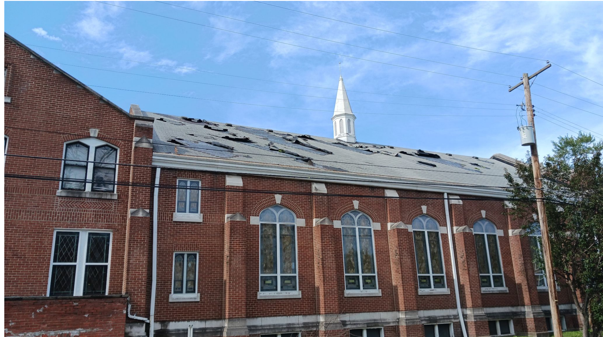
Roof damage at Calvary Baptist Church in Louisville after an EF-1 tornado on the 4th
