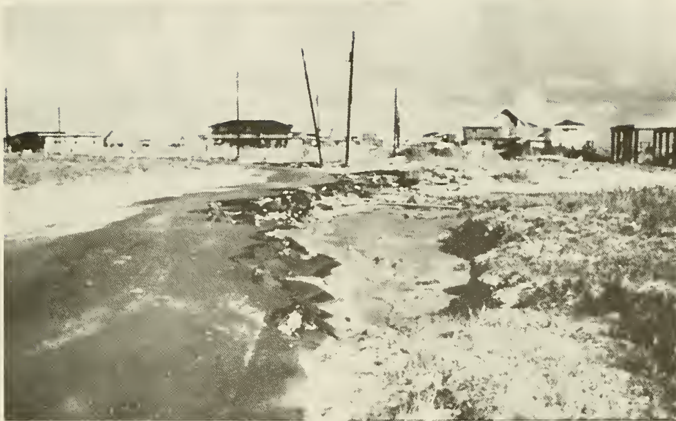
Photo 3. Damage to road on north side of Dauphin Island, looking west
