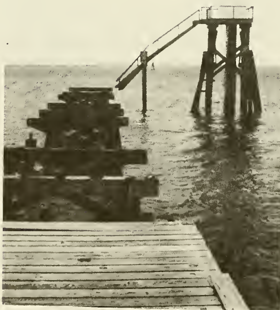
Photo 6. Pier damage at Pelican Point on the eastern end of Dauphin Island showing the NOS tide station where hydrograph of Dauphin Island (2) was obtained
