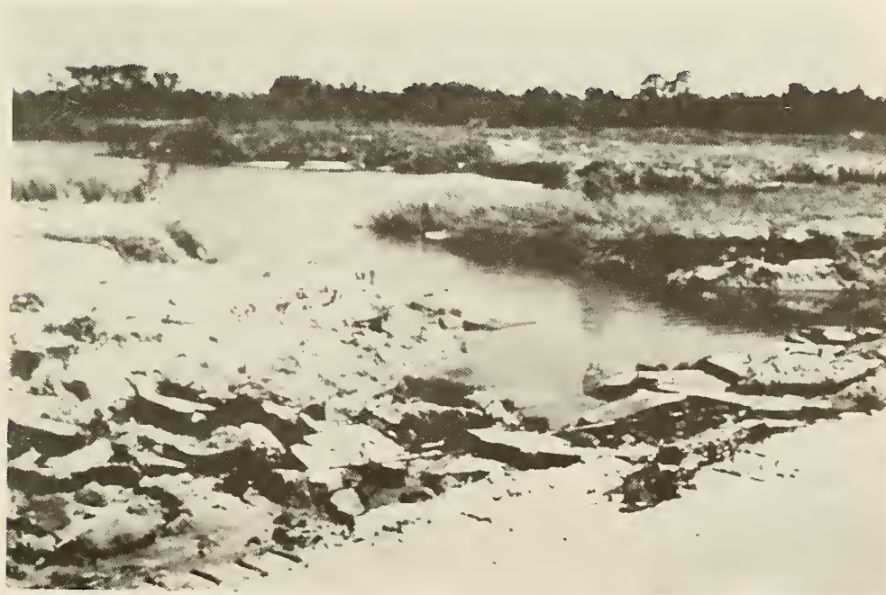
Photo 8. Evidence of overwash resulting in road damage in Ft. Morgan State Park, looking north
