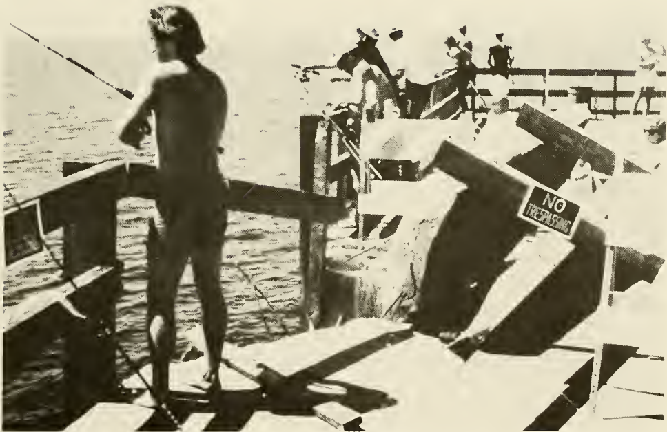
Photo 12. Damage to the decking of Dan Russell City Pier at Panama City Beach, Fla.
