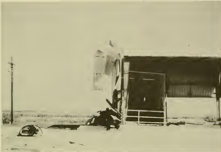
Photo 1. Damaged metal sheeting on Crain Brothers building, Grand Chenier, La.
