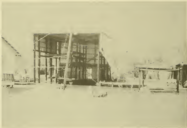
Photo 7. Damaged metal sheeting on a boathouse, Cyremont Point, La.
