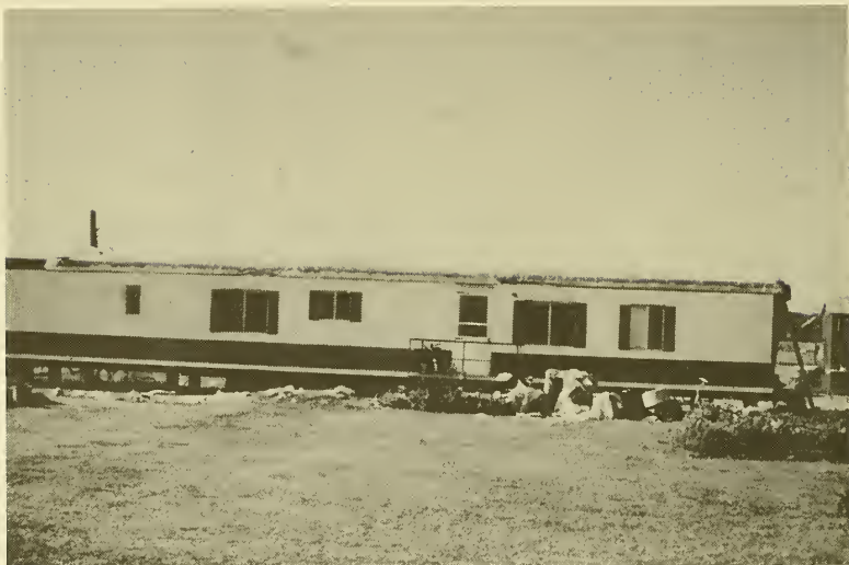
Photo 3. Mobile home roof damage near Pecan Island, La.
