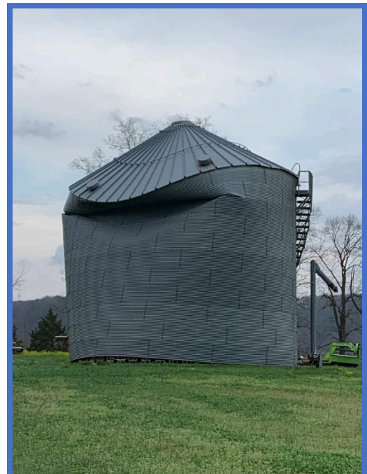
Blown-in Grain Silo in Rowan County Courtesy of NWS Storm Survey
