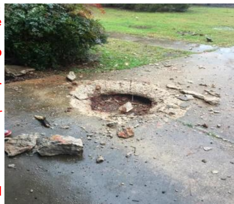
A lightning strike caused extensive damage to this driveway in Magee, MS. Photo by Chris Curlee
