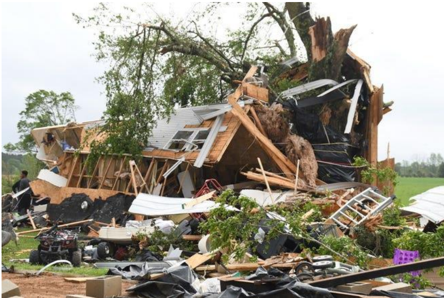
Mobile home destroyed by a EF1 tornado in Centreville, MS in April 2019. Courtesy of Trevia Reid.
