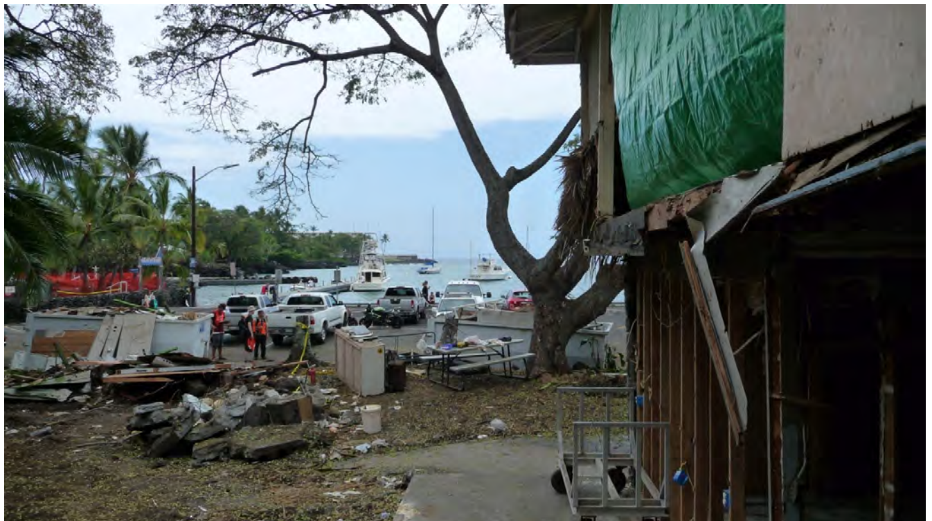
Figure B18b. View of Keauhou Bay outward from store. Wave reached top of vertical 2 by 4s (to right).
