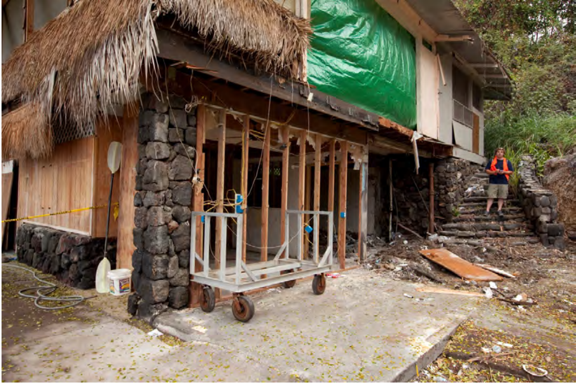
Figure B18c. Store-front walls breached by tsunami at Keauhou Bay. Wave reached top of vertical 2 by4s.
