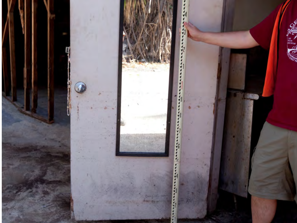
Figure B20b. Bar door with water-level line. Bar walls in background were breached by tsunami.
