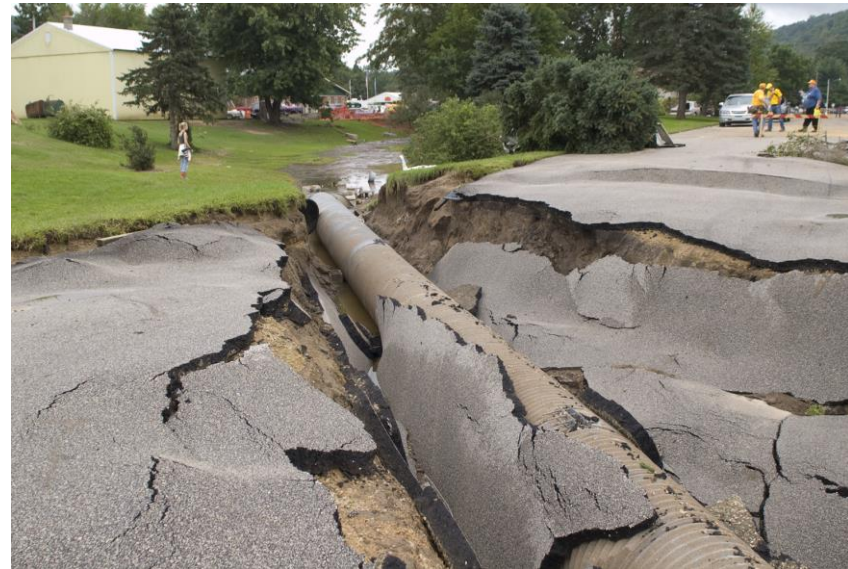
Minnesota road damaged by flood waters, courtesy of FEMA.
