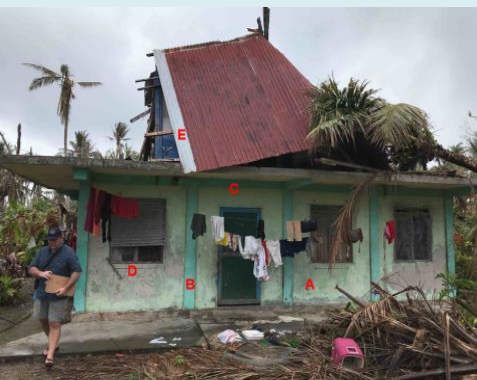
Concrete – CMU Walls strong - Metal Corrugated Roof damaged by Typhoon Wutip
