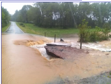
Right: Part of road washed out in Iredell County, NC during Hurricane Michael.
