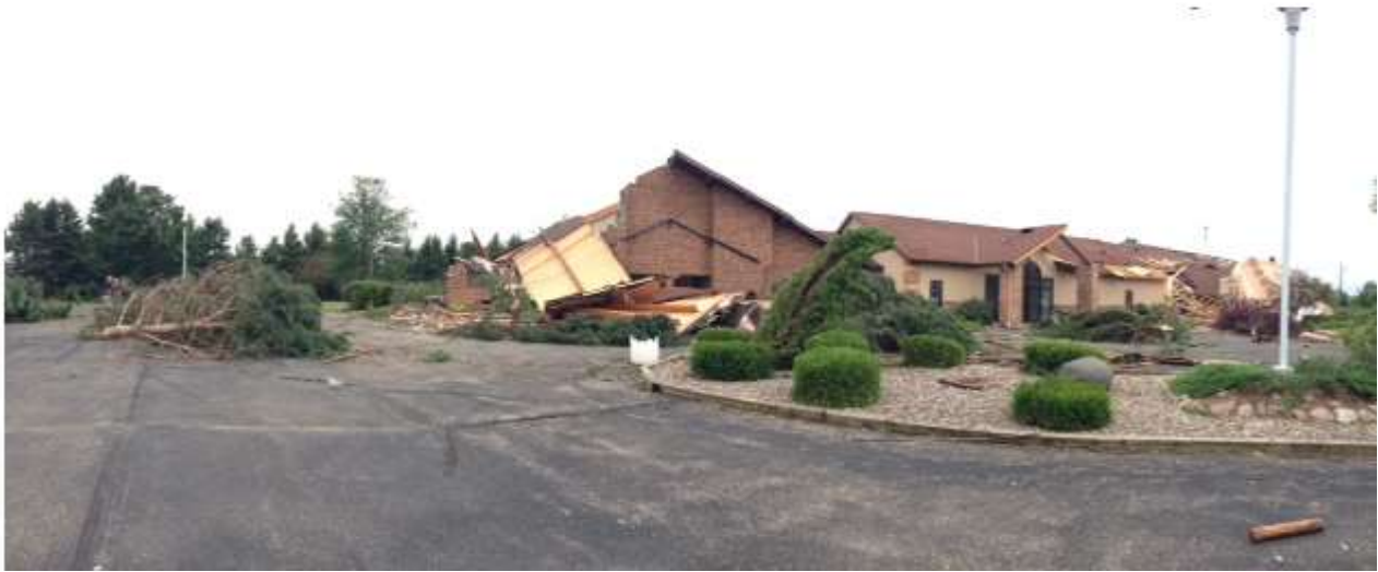
Figure 1: Church (southeast New London) damaged by a tornado. Peak winds were estimated at 115 to 120 mph.
