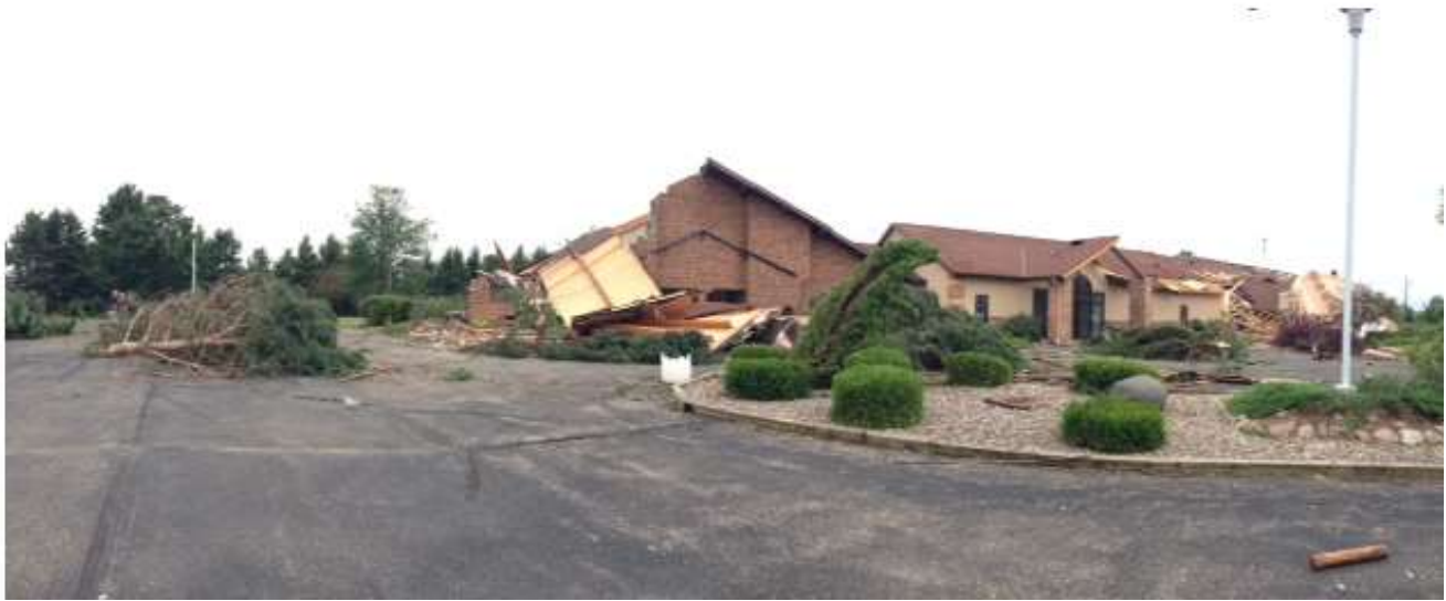
Figure 1: Church (southeast New London damaged by a tornado. Peak winds were estimated at 115 to 120 mph.
