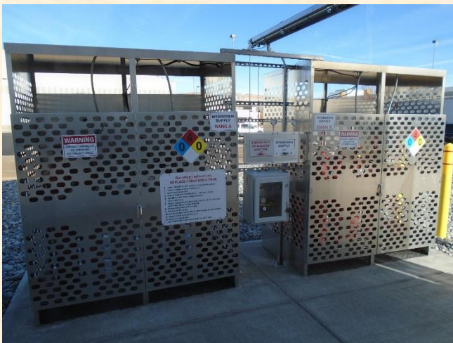
Image 1: Bank A and bank B cages that housed the hydrogen tanks and delivered hydrogen gas safely from the outside of the inflation shelter to the inside using the HISS. Credit: John Kyle
