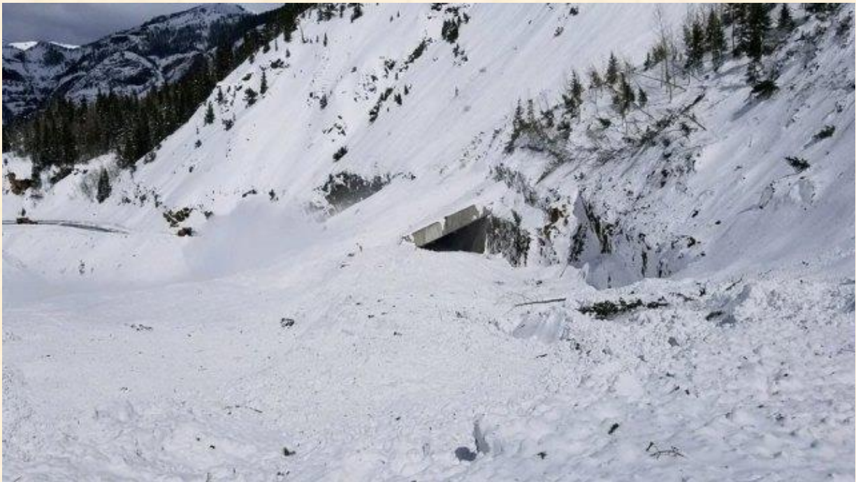
Image 2: 40 to 60 feet of snow brought down from avalanche mitigation over Highway 550 in March 2019 over Red Mountain Pass, filling the Snow Shed on Highway 550. Credit: CAIC/CDOT
