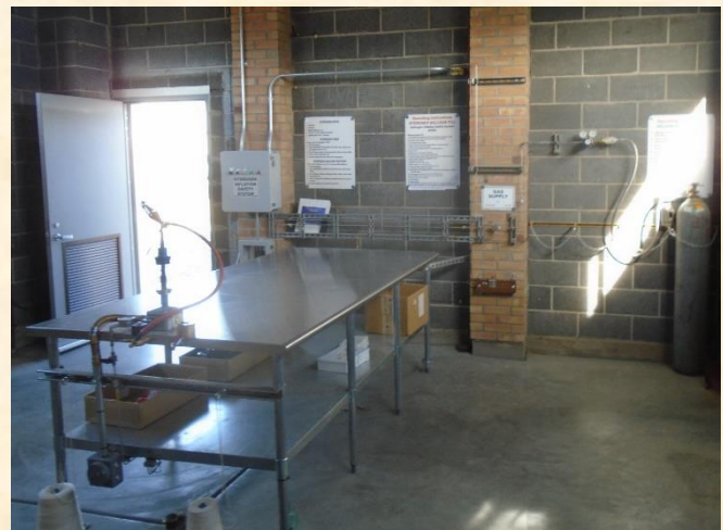
Image 2: Inside the inflation shelter showing the redesigned upper air configuration using the HISS. Backup helium option to the right of the image with ability to switch back and forth between hydrogen and helium safely. Credit: John Kyle
