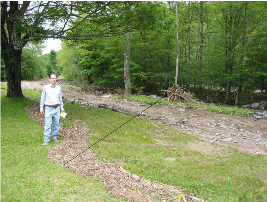
Figure 16. Berry Brook indirect discharge location. Black line drawn in to show water surface elevation consistent between right bank high water mark and in-channel debris.
