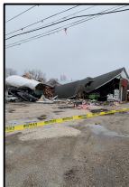
Figure 3: Tornado Damage Surveyed in Colona, IL
