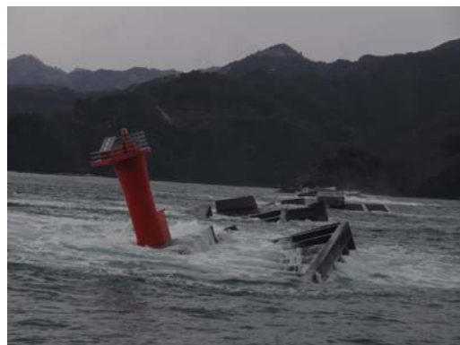
Photo 7 Damaged caissons of Kamaishi Breakwater
