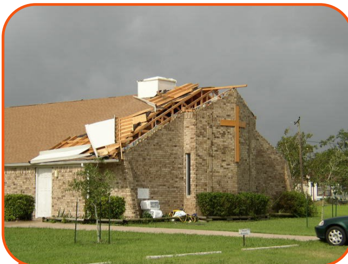
Damage to church in Port Lavaca
