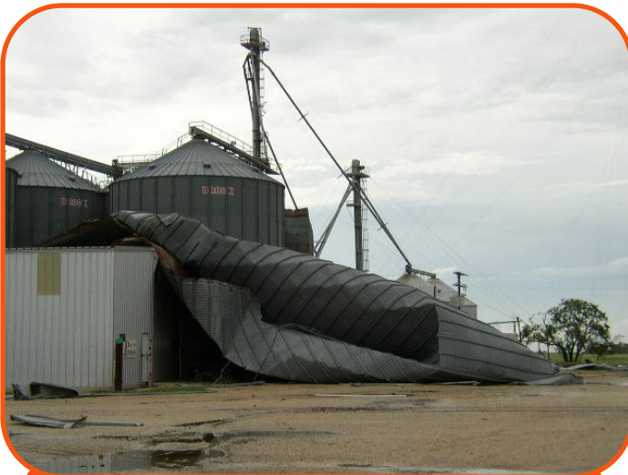
Damage near Long Mott
