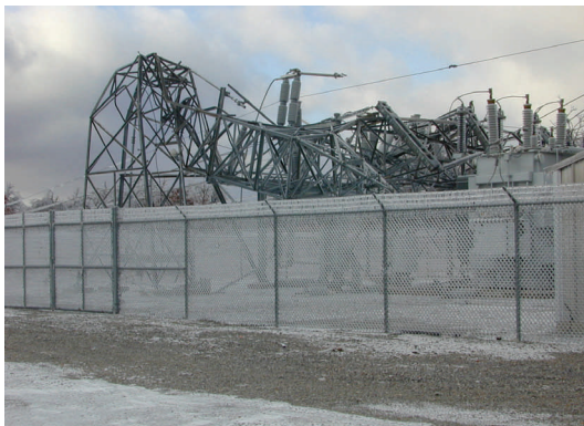
Above: A Transmission line tower crumpled from the weight of ice during a 2007 storm in Oklahoma.
