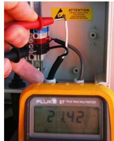
Figure 7.6 Solar Voltage at Terminal Block
