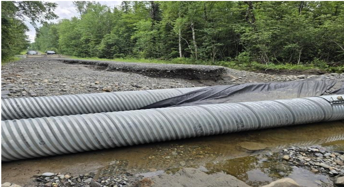
Bates Rd. Abbot. Underneath taking of this picture there are two 5' culverts that may have potentially failed. Water receding
