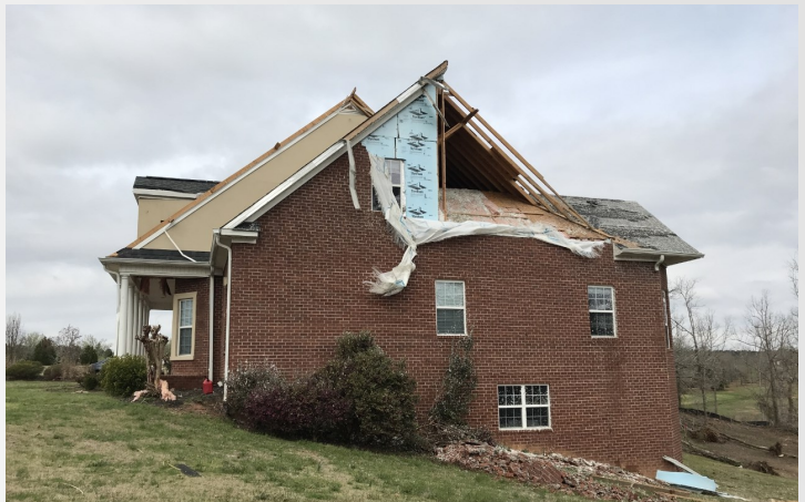
Roof damage to home from EF2 tornado in Evans, GA
