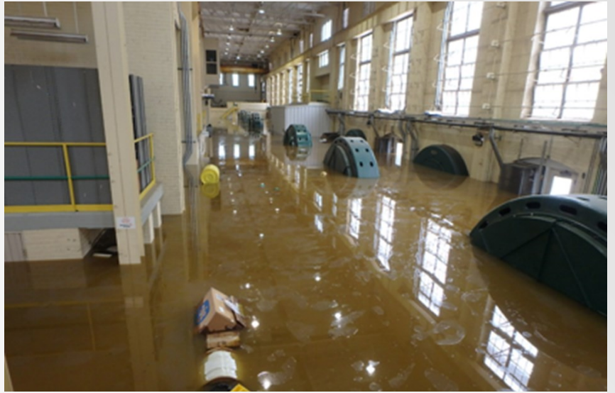
View from inside the Blewett Falls Dam powerhouse while it was flooded from Hurricane Florence
