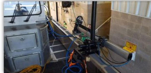
Figure 4: MIST installed on a trailer-able aids to navigation boat.
