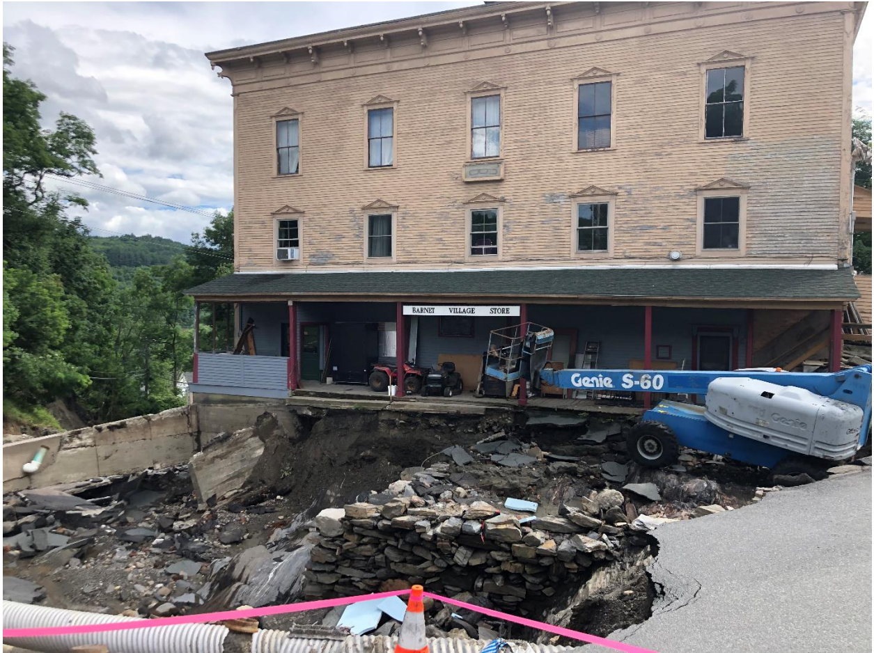
Figure 6: Catastrophic Flooding in Downtown Barnet.
