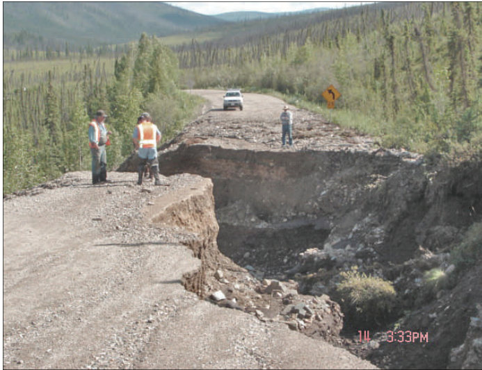
Taylor Highway at Milepost 81, near Walker Fork Campground A culvert washed out, leaving a hole approximately 20 feet deep and 60 feet wide
