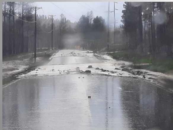
July 29 Gavilan Creek flood Photo courtesy USFS Baer Team
