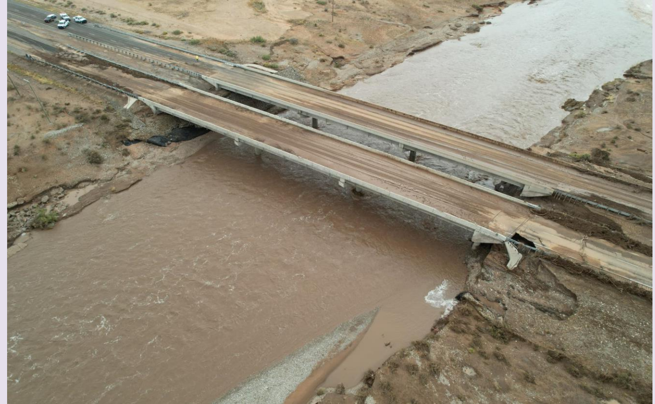
Flood Damage to HWY 285 Bridge over Rio Felix Near Dexter 10/20/2024 – Courtesy Craig Schinnerer
