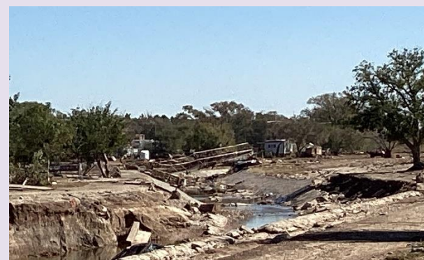
Canal damage from Roswell Flood – Courtesy Scott Overpeck
