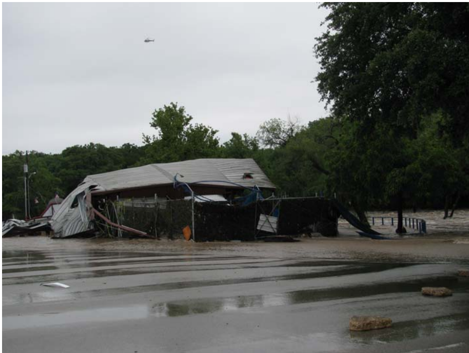
Photo 2, Building damage near the Gruene River bridge
