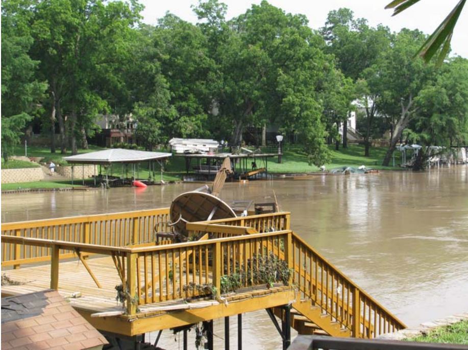
Photo 15, Debris on top of decks below Lake Dunlap
