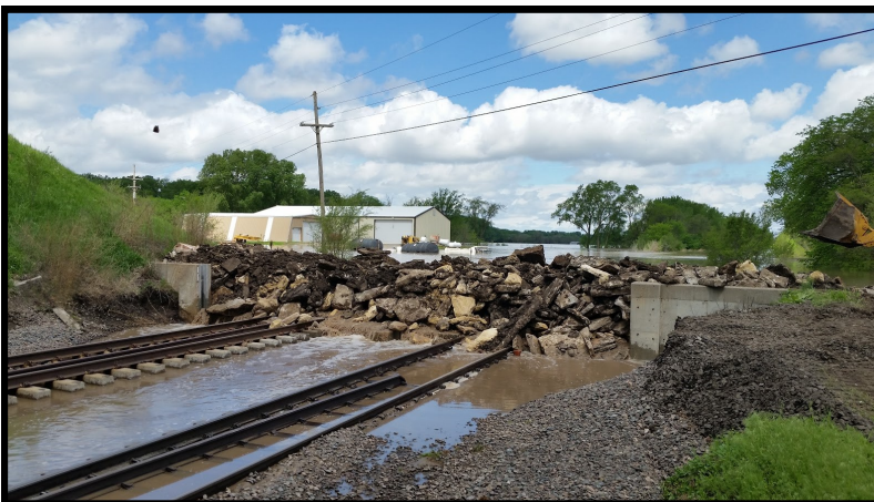
Flooded railroad tracks near Fairbury. Photo courtesy of Jefferson County EM.
