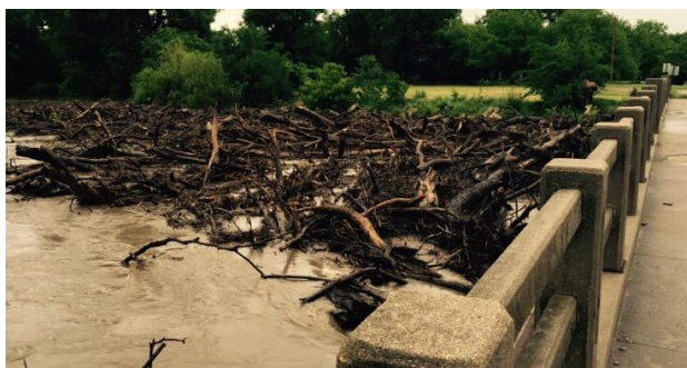
Flooding along the Cottonwood River near Florence, due to several bouts of heavy rain across the region during the second half of May.
