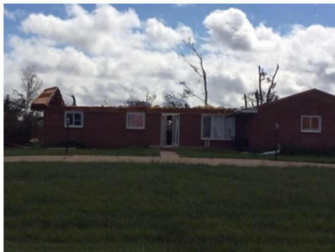
Tornado damage from the May 6 tornado northeast of Webber, KS. NWS storm survey photo.
