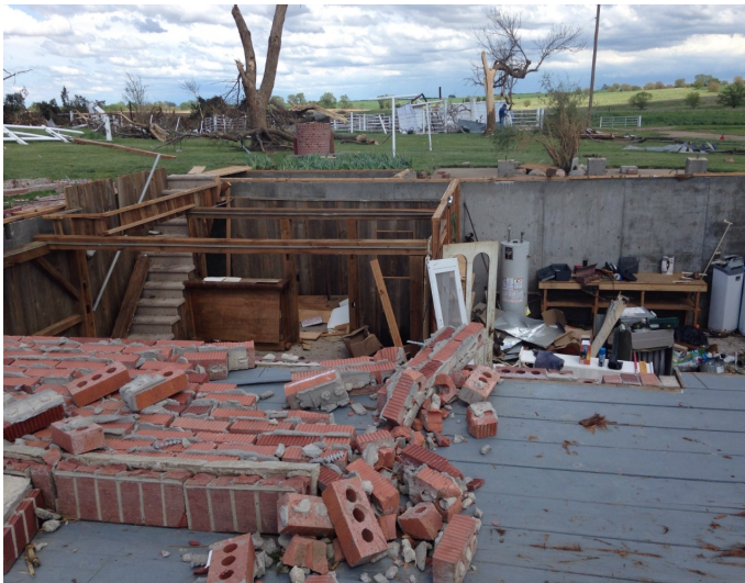
Home destroyed near Munden, KS on May 6th, 2015
